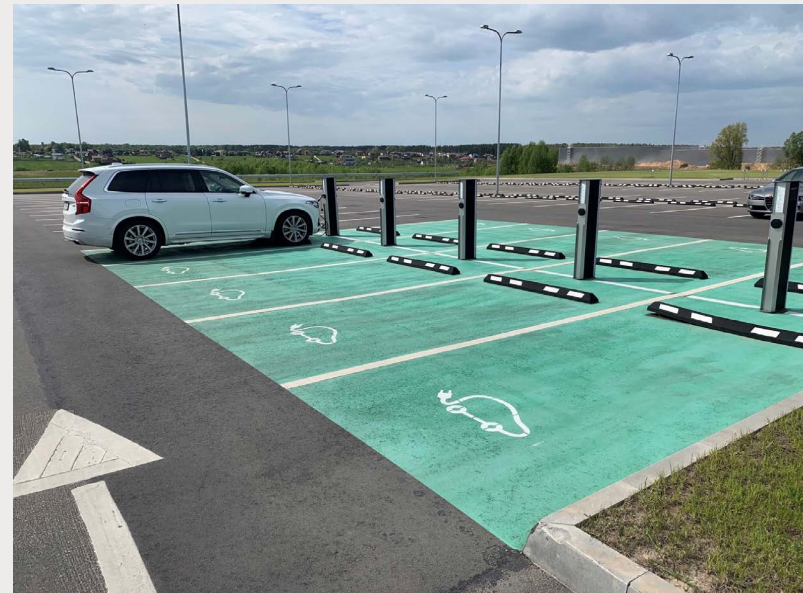
Electric car charging stations
